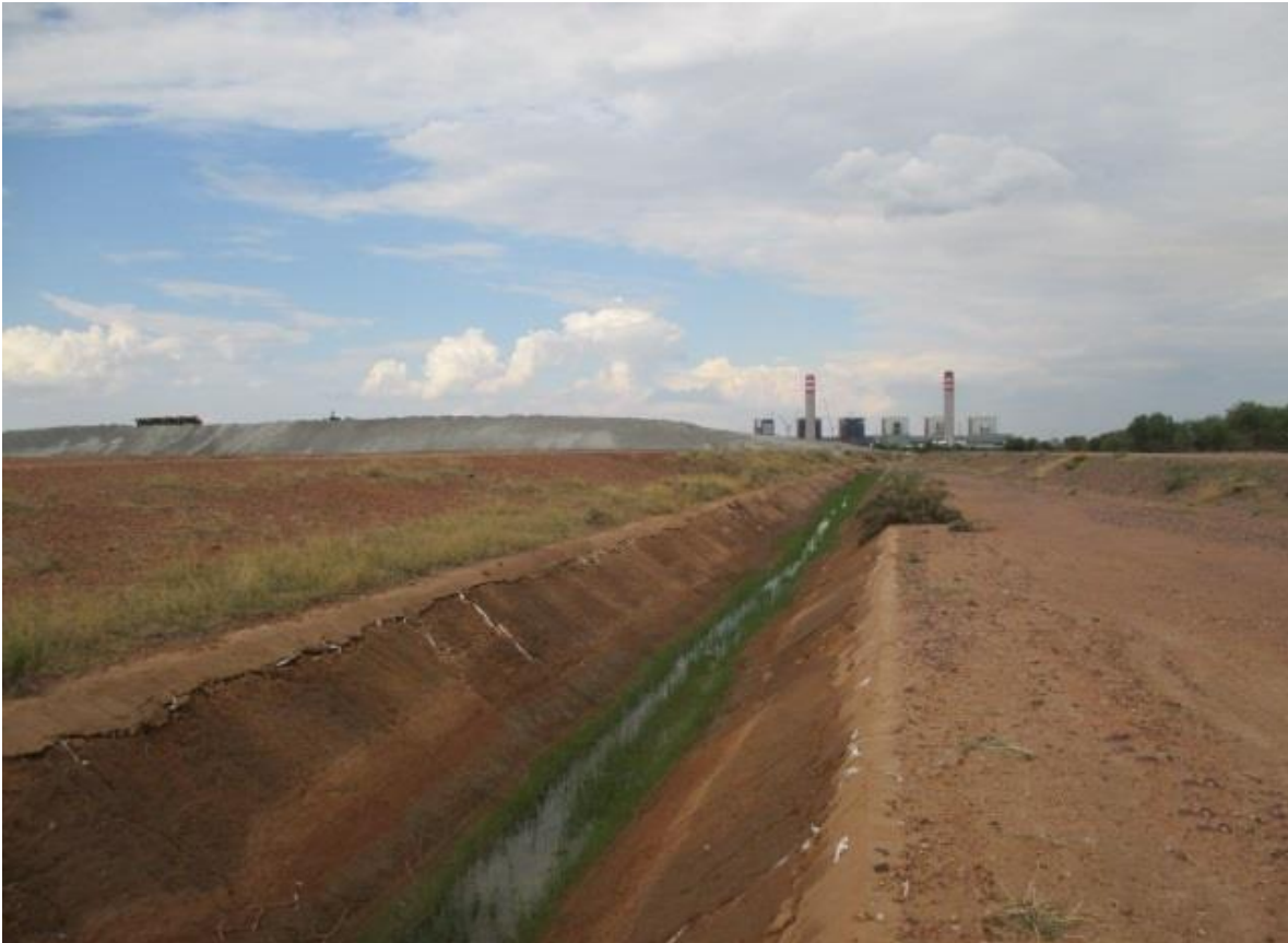
Figure 11: Concrete-lined dirty water containment drain alongside ADF at Medupi
